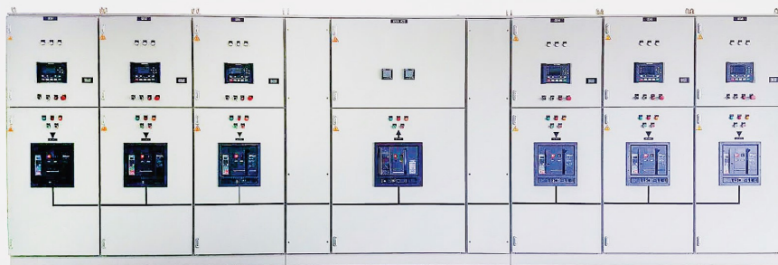
GCP 7500A PROJECT : POWER PLANT (MYANMAR)
